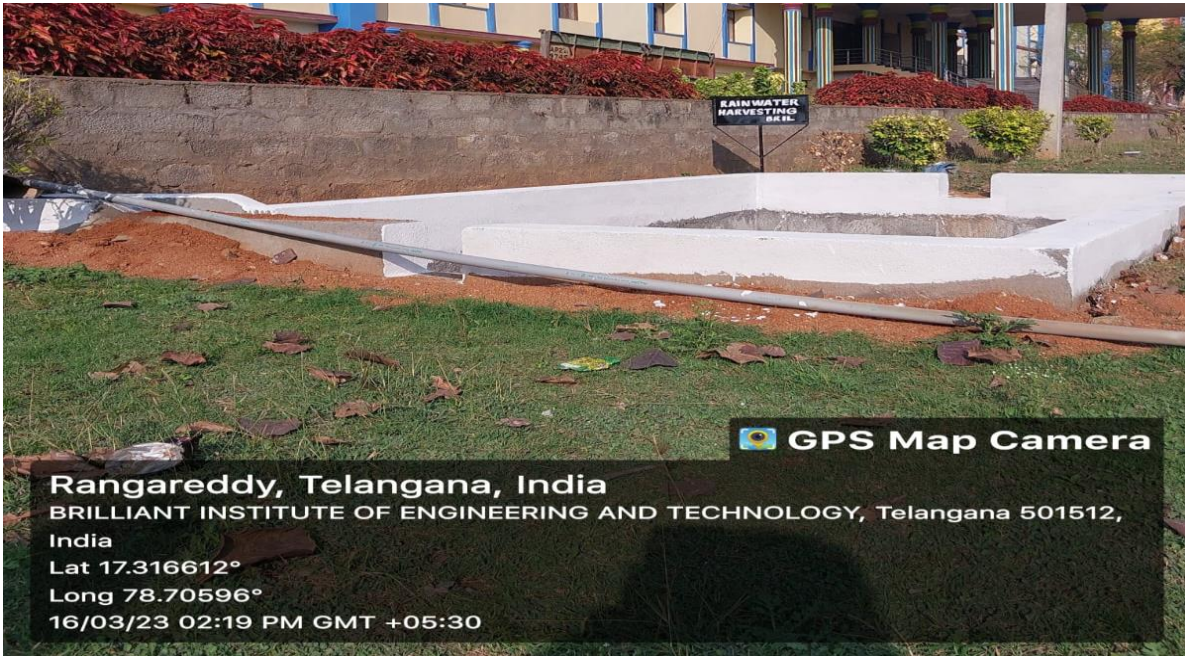
Rain water harvesting pit.
